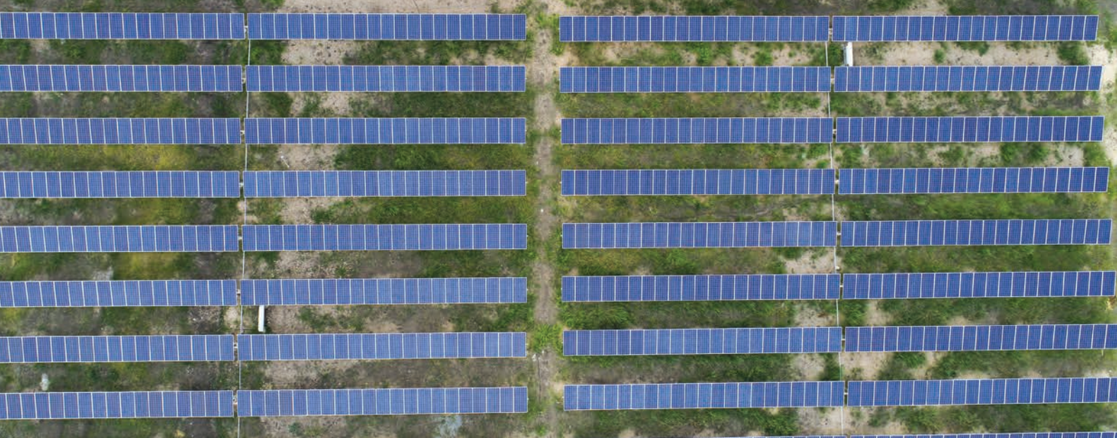
Fig. 1.22. Solar farm near Raichur, Karnataka
